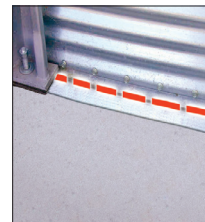
Sill Plates and ground level water seams
