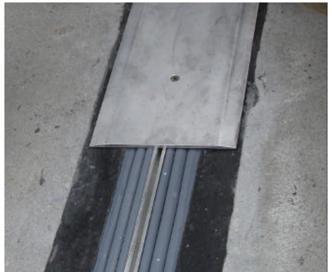
SJS SYSTEM installed with EMSEAL elastomeric nosing material in blockouts on each side of joint gap.
