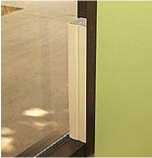
ABOVE: QuietJoint SHG installed between window glass and end of wall partition. The third silicone side faces the glass. The silicone color of this sample is Dow 790 Sandstone and was chosen deliberately to contrast with the surrounding colors. A "Bronze" color choice would allow the QuietJoint to coordinate completely with the bronze mullion.
